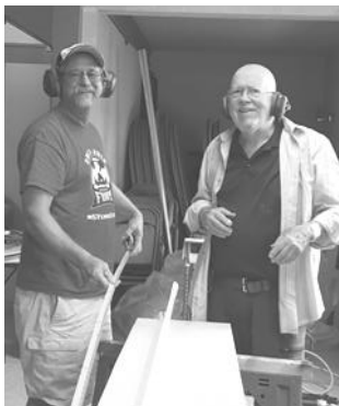
Brad Copeland and Tom Safford working on a new storage door in the Fellowship Hall. "Measure twice; cut once!"
